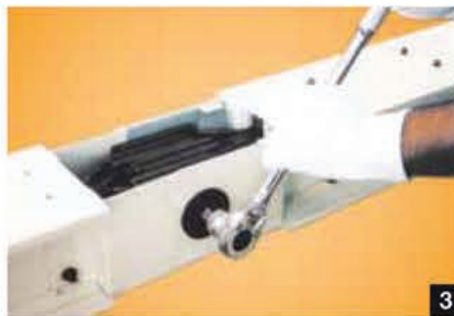
Tighten the "MF" nut by special ratchet wrench till the neck part of the nut is broken and locked.
